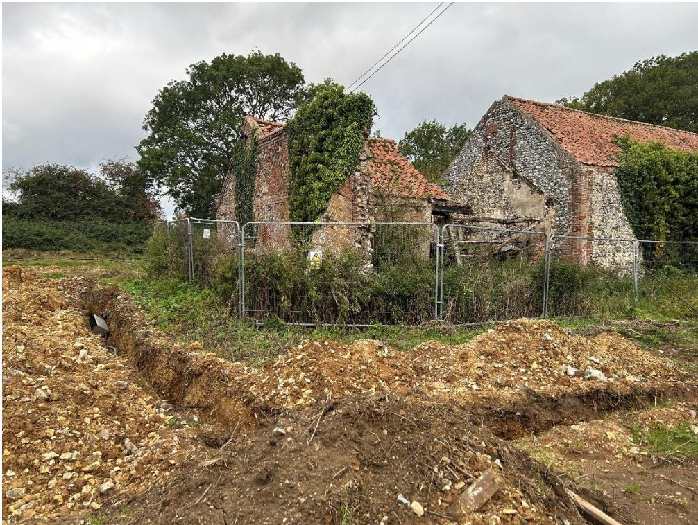
Plate 12-6 Derelict property at Abstraction 6/33/58/*G/0248
