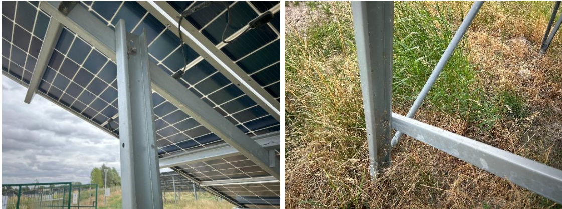
Plate 12-15 Indicative thin racking system driven into ground
